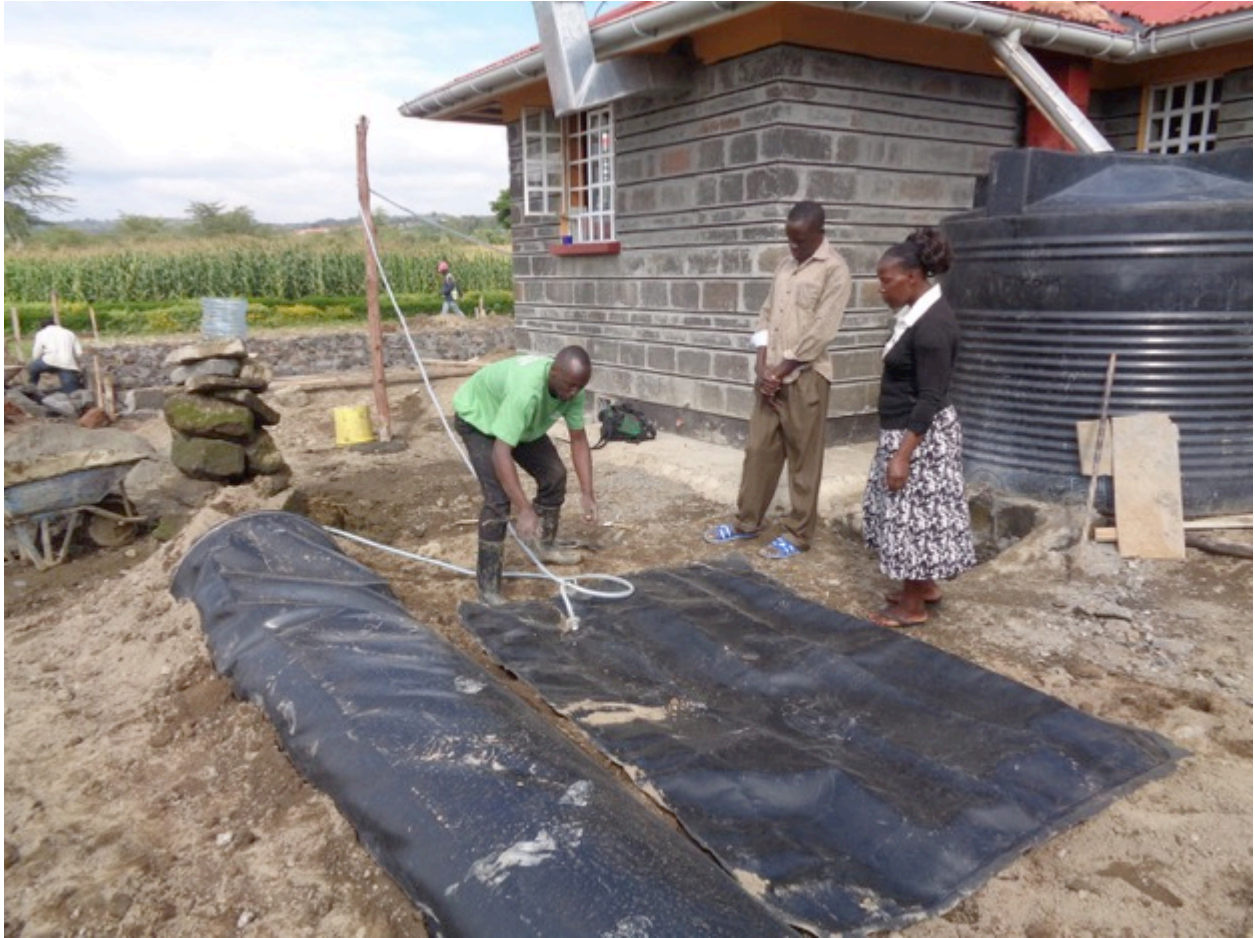
Peter Langat from Jomo Kenyatta University while setting up the home gas installation
